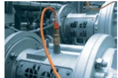
Accelerometers type VSA are connected to VSE units to monitor critical components of the process (pumps, motors, agitators).
