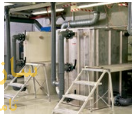
Level measurement in a water treatment plant
