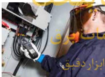
Analyze Power-related Issues
