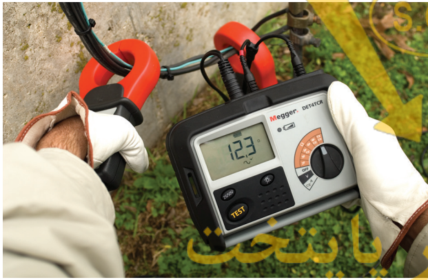
Model DET4TCR2 shown performing the stakeless ground testing method using only clamps.
